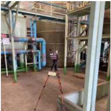
Area : WasteWater Treatment
